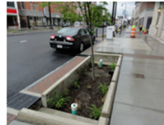
Bioretention planter in urban downtown setting.
