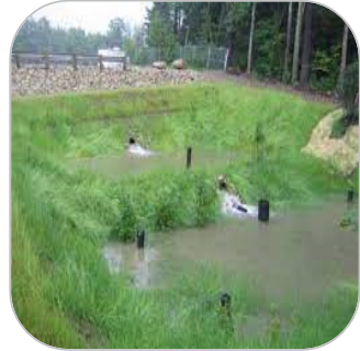
Stormwater Wetland BMPs
